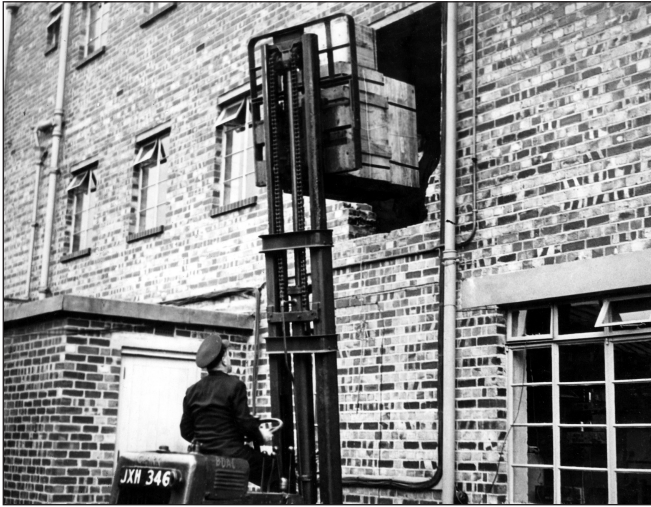
Figure 4. Equipment was hoisted by a fork-lift through space opened by knocking out a side window.
