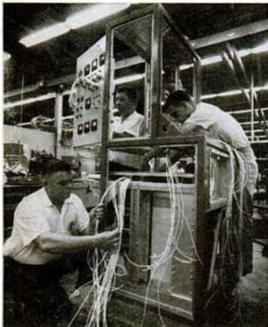
POWER-SUPPLY CABINET , being wired above, feeds two transmitters that simultaneously broadcast different programs from TV plane.
